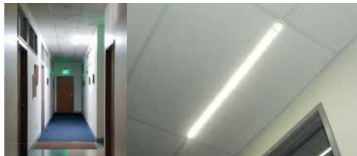
Power outage - emergency LEDs activated
